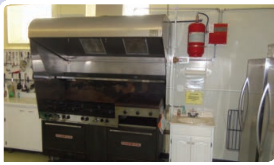
A new fire suppression system has been installed over the hall kitchen range at St. Paul the Apostle in Calumet. This fully licensed kitchen is used often in service to parishioners and community with weekly bingo concession, funeral luncheons, fall festival, and more.
